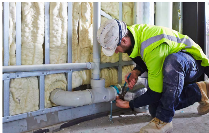
7. SERVICES CONNECTIONS MADE
