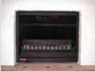
Existing Jetmaster wood fire
