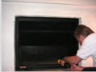
Logpan removed and a 25mm hole is drilled on the RHS of the firebox.
