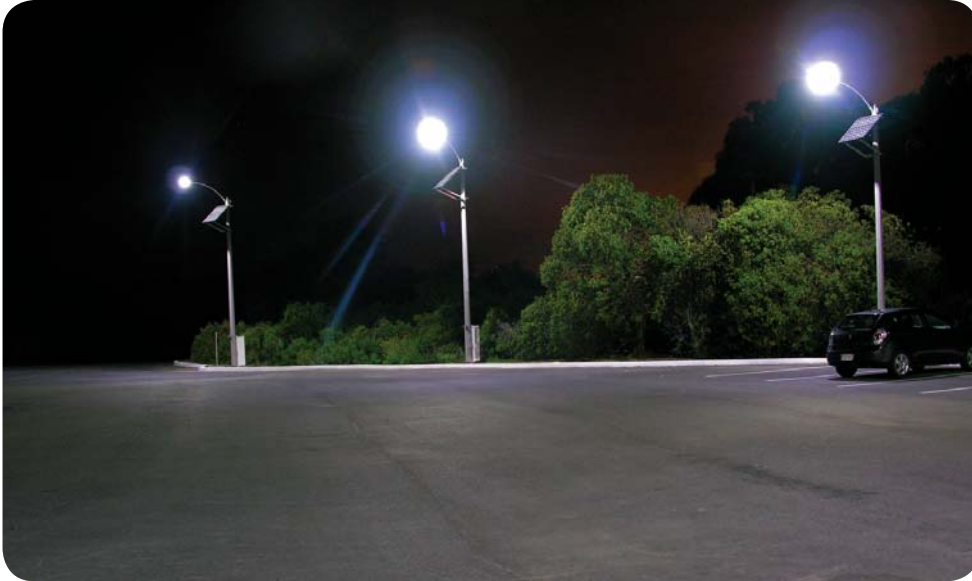
Carmanah EverGEN™1520 Solar LED Lighting Solutions installed at a California Energy Facility
