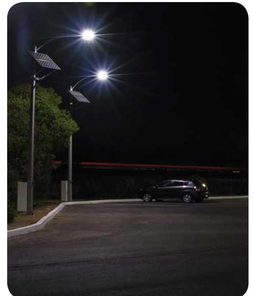
Carmanah EverGEN solar LED lighting solutions feature BetaLED™ fixtures and are fully compliant with Dark Sky Association guidelines and IES full cutoff standards.
