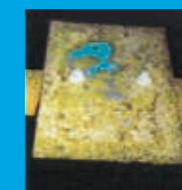
Alkyd coating: Covered with rust
