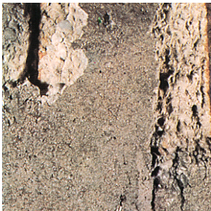
1.1 Visible effect of carbonation on concrete
