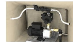
Pump installed with rain/mains changeover (sits behind door)
