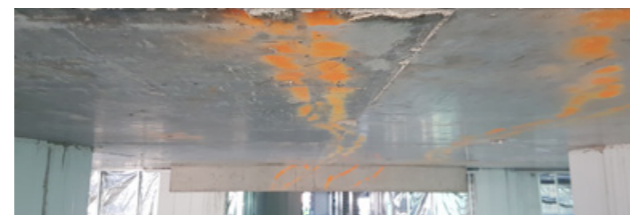
Formwork residue and concrete debris often present uneven fixing surfaces which are not made good prior to wall installation.
