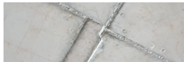
Misaligned formwork was identified as a contributing factor to tension in internal framing.
