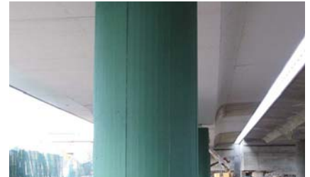
Principle 9, method 9.1 Masterseal coatings applied directly on the concrete to protect the underlying reinforcement.
