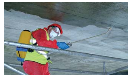
Principle 9, method 9.1 Corrosion at the cathodic areas of the reinforcement is inhibited by the use of Protectosil CIT.
