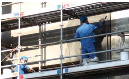
Principle 3, method 3.1 Emaco repair mortars: Emaco Nanocrete R4 / R3 / R2 / FC hand applied.
