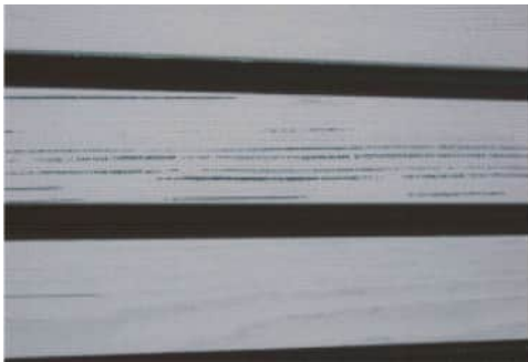
Deep grooves and cracks
