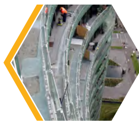
High rise residential balcony failures
