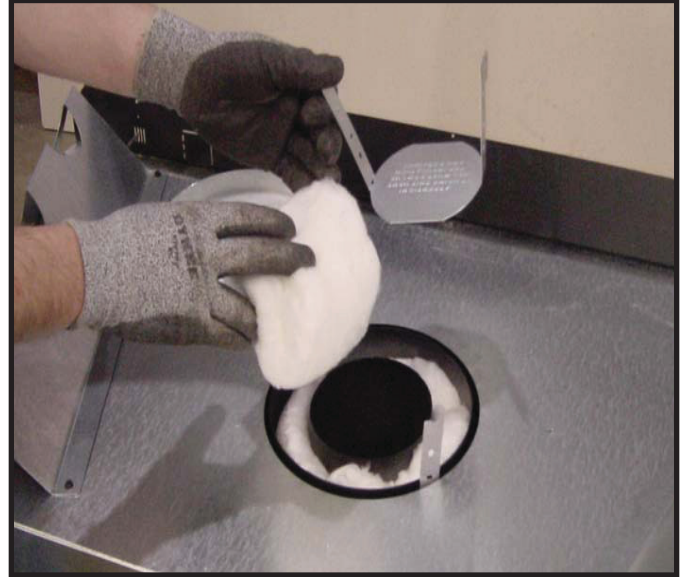
Figure 9.4 Remove the insulation basket and white insulation from the center vent pipe.
