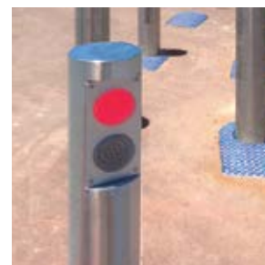
Above, use of traffic light bollards at a busy access point and left, exterior cabinet with compressor and logical controller.
