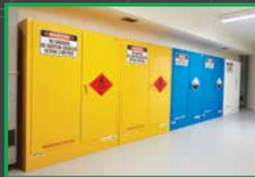
E. SECURE CABINETS FLAMMABLE CABINETS CORROSIVE CABINETS
