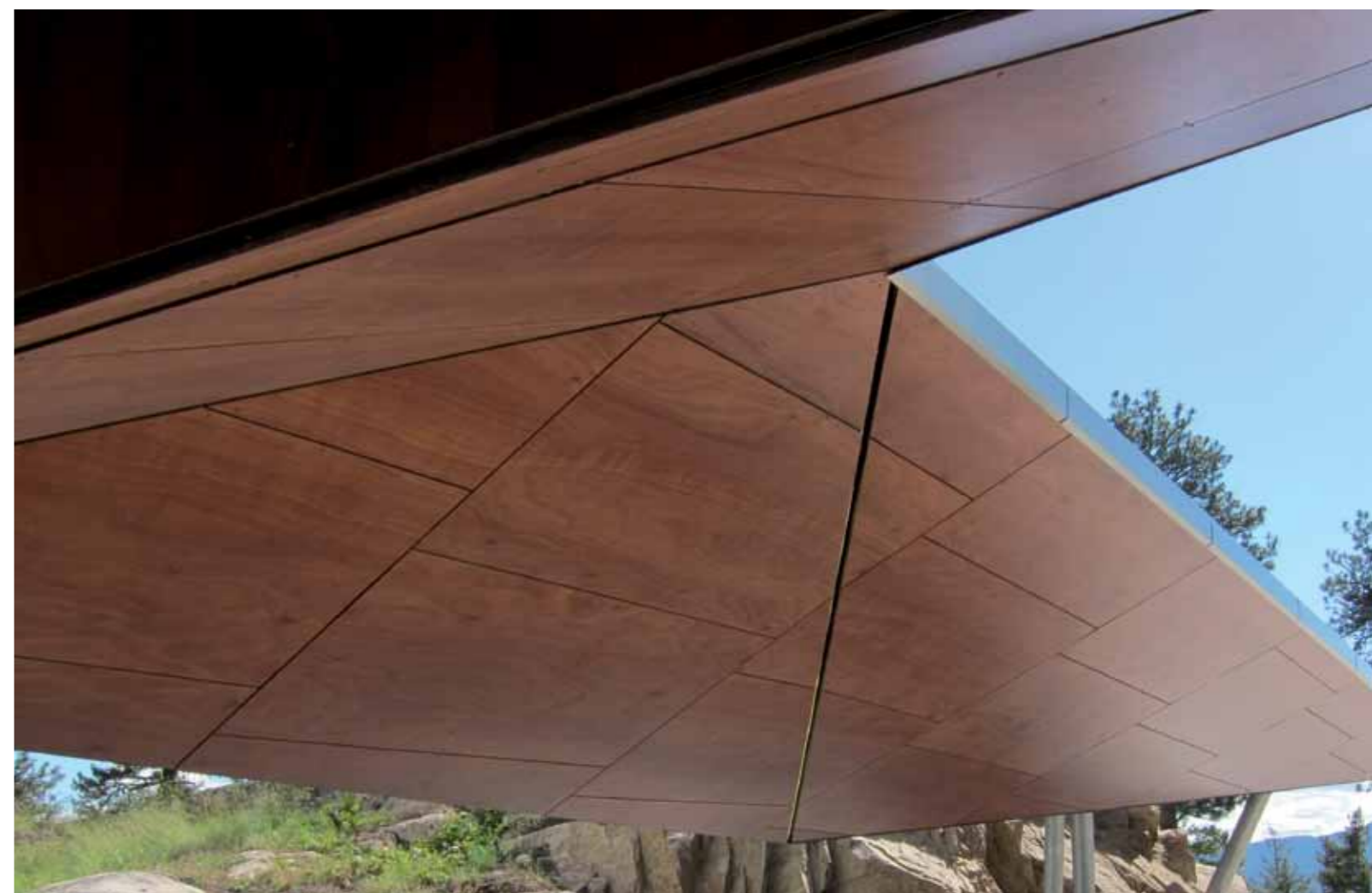
SUSPENDED CEILING: VISIBLE FIXINGS
