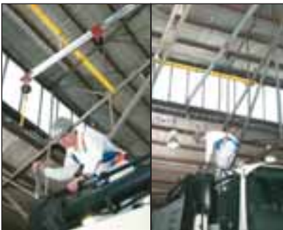
OVERHEAD INTERNAL SYSTEM FOR MAINTENANCE
