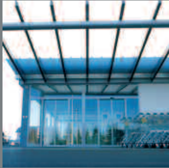
→ Emergency opening by electrical energy accumulator (BAT)
