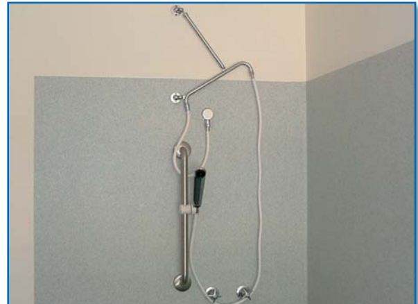
Picture showing # ClevaKit010 installed at the Independent Living Centre.
