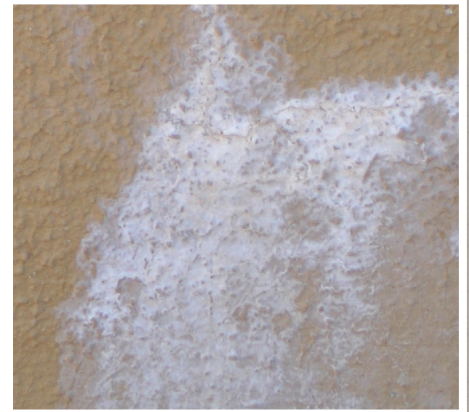
Eliminate unsightly efflorescence
