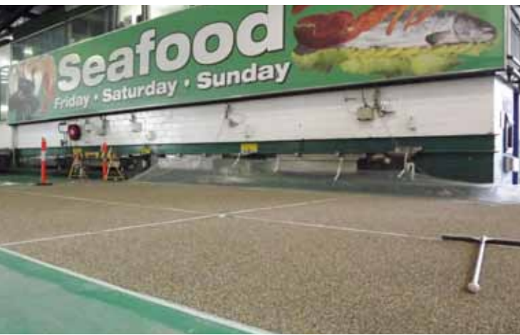
Installing a very heavy duty anti-slip system at the Sydney Fish Market
