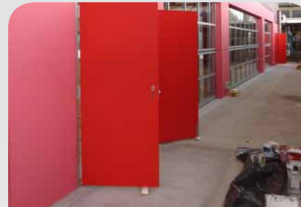
Application of the Envirothane 8480 system in progress on multiple surfaces at a school in NSW.
