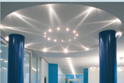
Foyer lighting solutions
