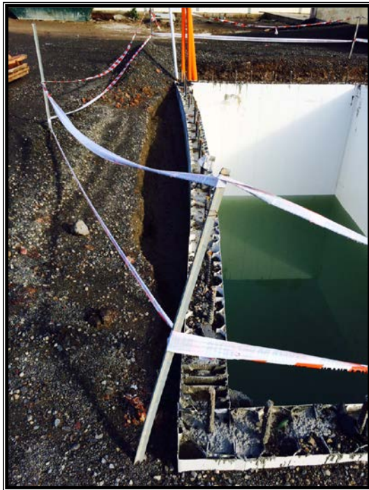
Photo No: 1 – Shows Displaced Wall
