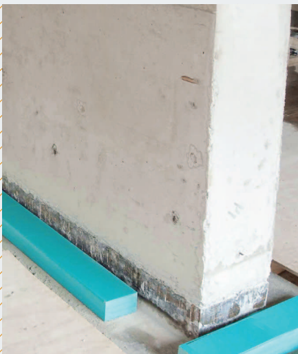
Detail of the pointwise support of the Mezzanine floor. Bearing dimension customized according to given performance criterias as well as specific loading.
